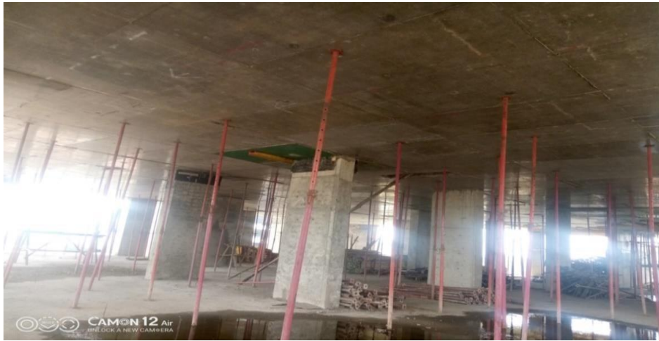
Figure4.1 project one conventional slab after 45 days casting concrete
