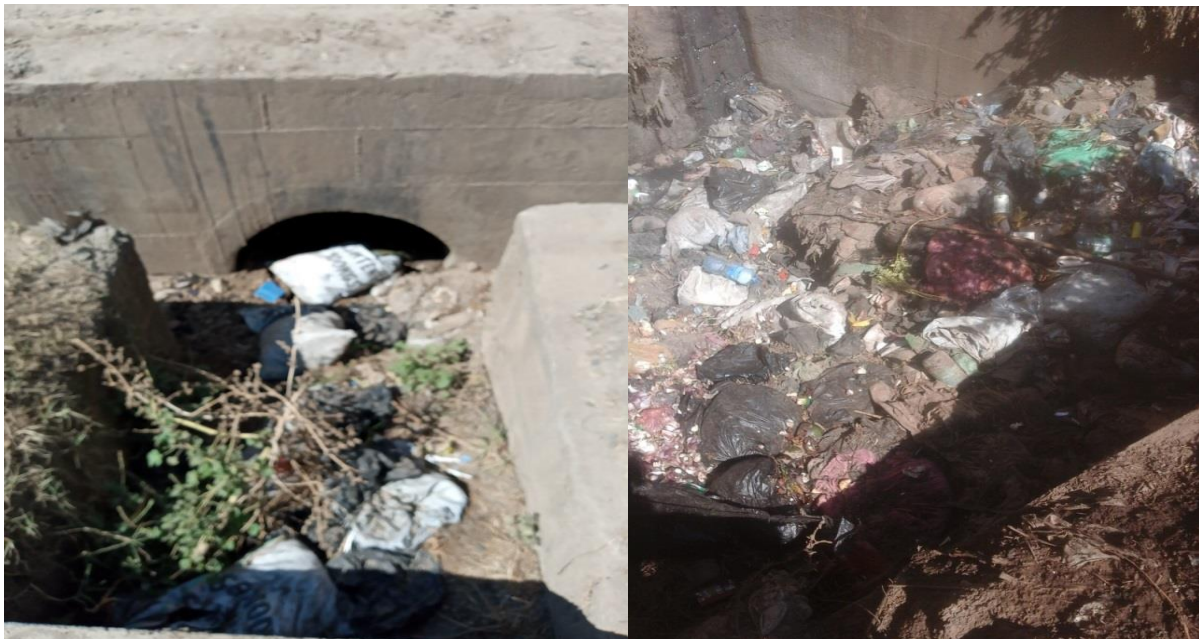
Fig 2.5 Solid wastes filling pipe culvert and reduce the flow capacity
