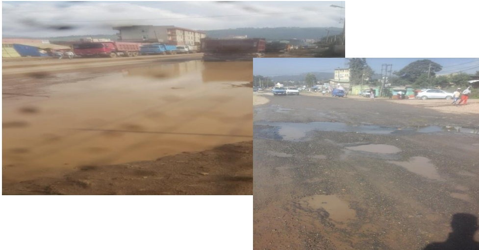
Figure 4.10 Severe failures of road due to water ponding on surface (Maskerem Hotel)
