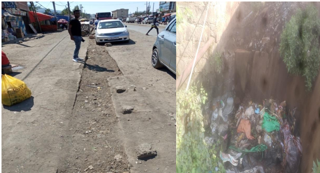
Figure 4.7 Solid waste dumped in to drainage ditches & culvert
