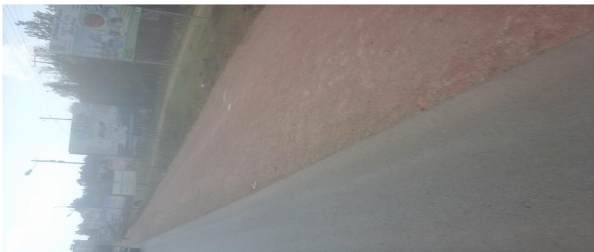
Figure 4.11 No side drainage ditch from Was fuel station to Nock fuel station
