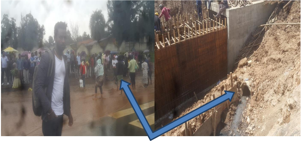
Fig 4.5 Existing Road Drainage Structures Problem at Furi Area
