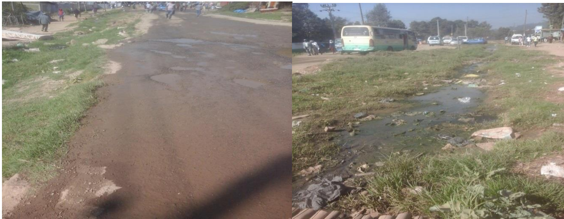
Figure 4.9 Drainage ditches blocked with grasses, silt, debris & sand accumulation
