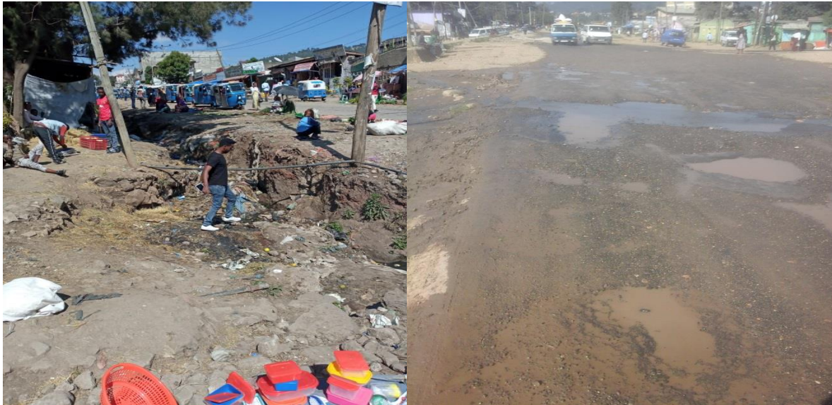
Fig 2.4 Road cracking due to failure of side ditch
