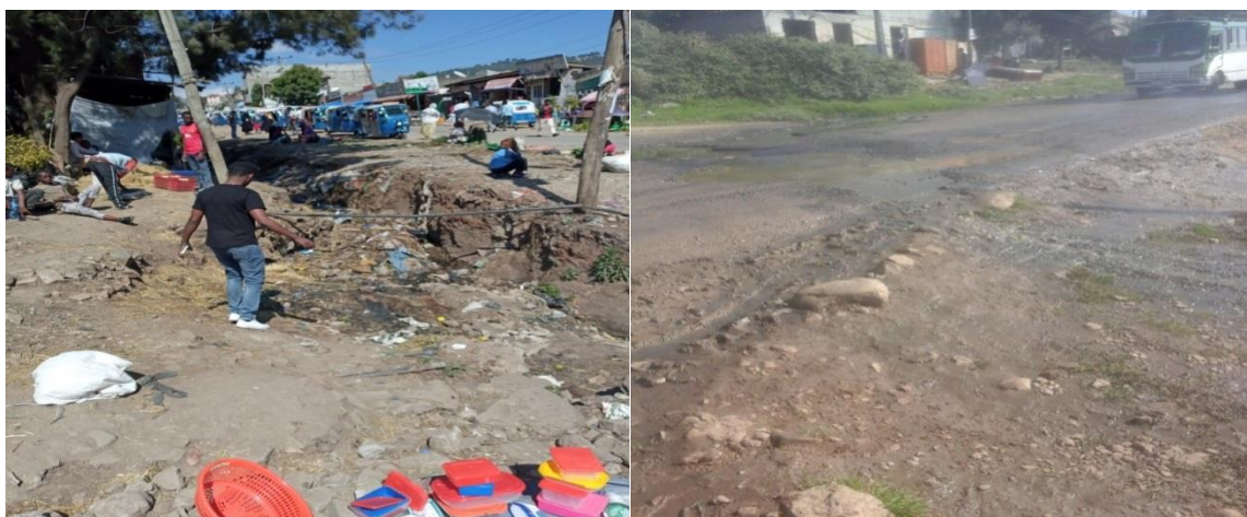
Figure 4.8 Failure of ditch and pavement distress.
