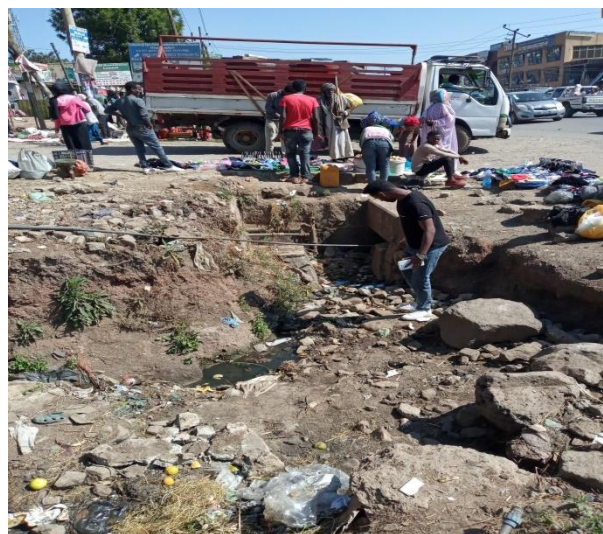
Fig: 2.3 scours of culvert at inlet discharge
