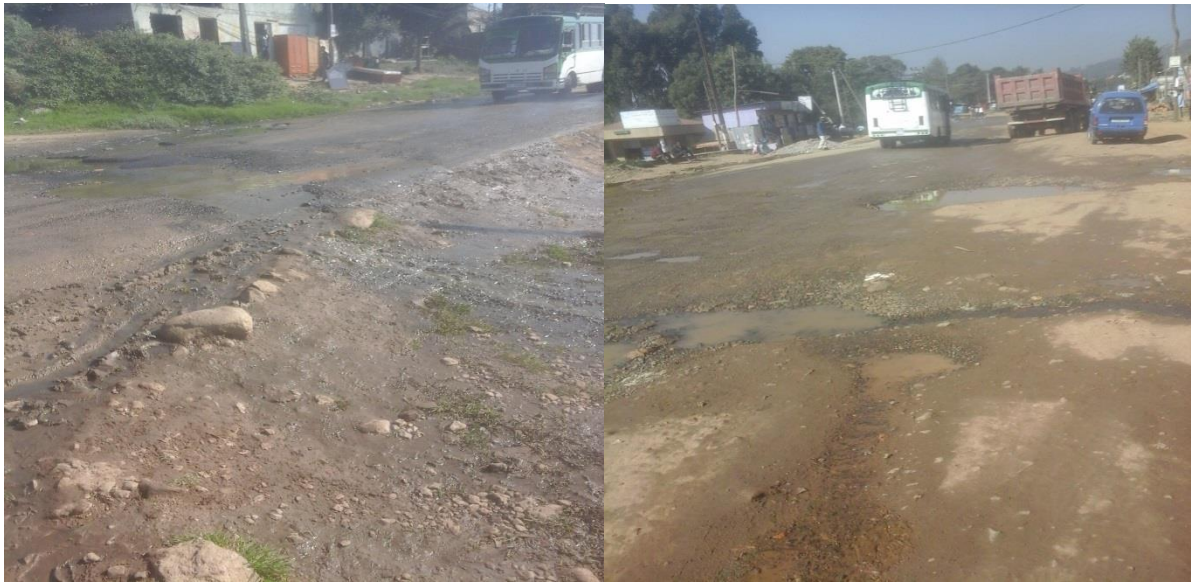
Figure 4.12 Road edge failure and pond of water
