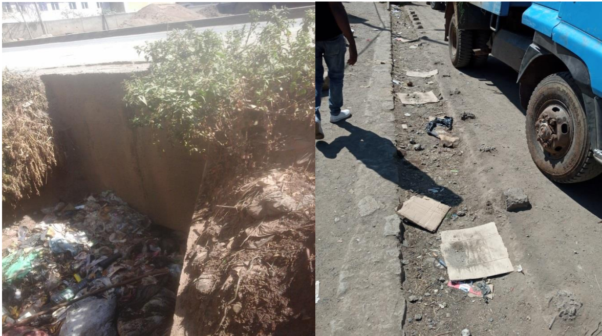
Figure 4.13 Culvert and roadside ditch discharge points totally blocked with refuse dumps
