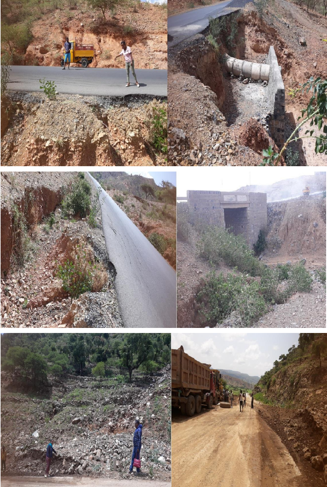
Figure3. 2 Many Cracks on road surface, ground subsidence and Slope instability
