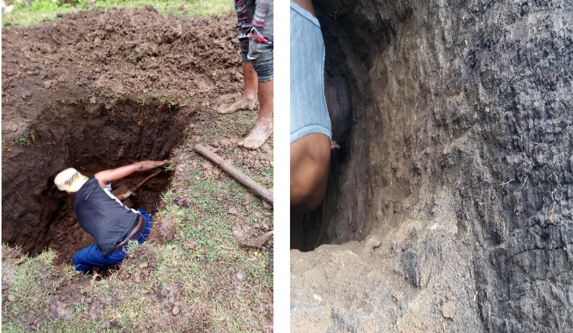
Figure 17 Excavation of test pits during sampling (Source: photos taken during test pit excavation)
