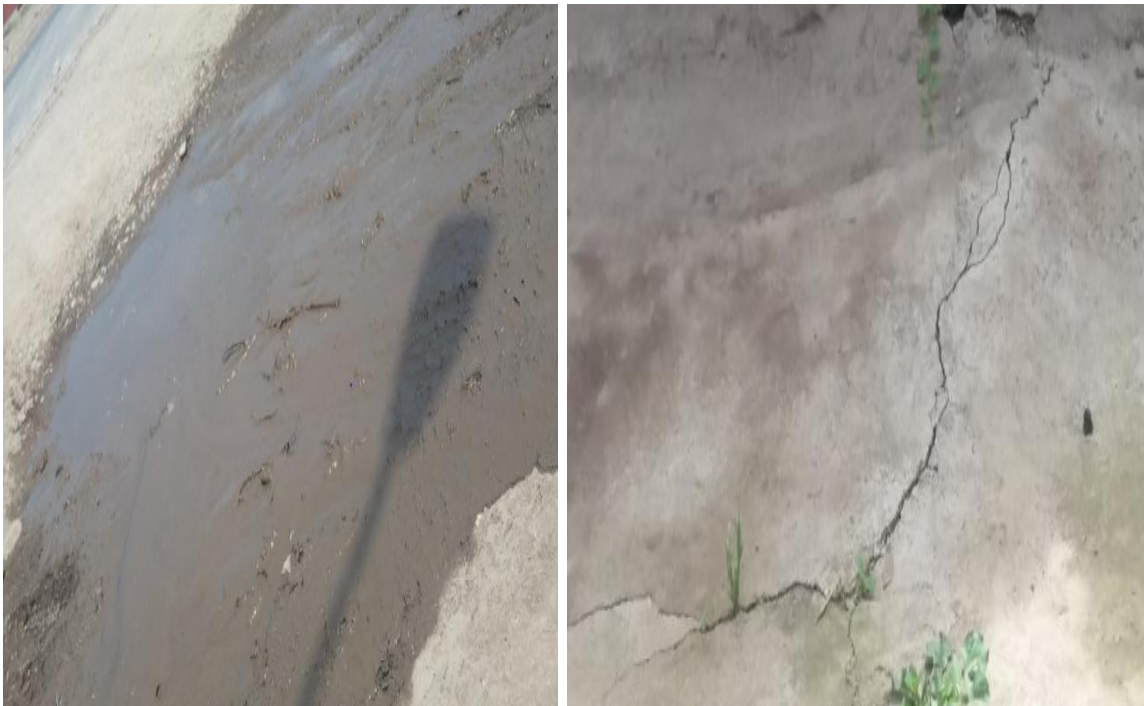
Figure 1 Problems that occurred due to expansive soils in Bishoftu
