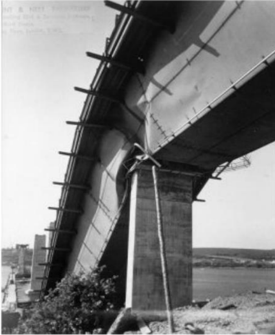
Figure 1-3 Failure of plate girder due to web buckling
