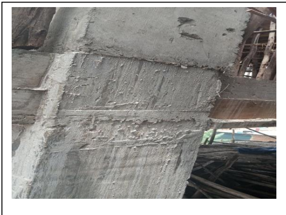
c) Poor construction joint
