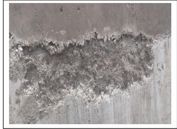
b) improper termination of formwork
