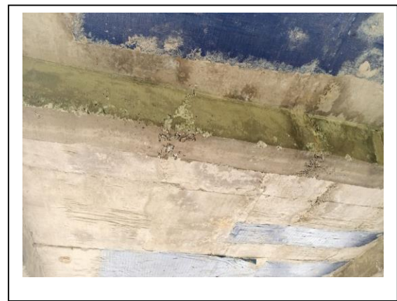
d) formwork stuck on concrete surface
