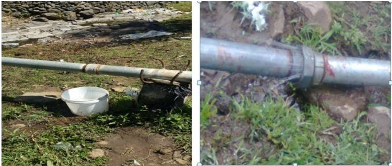
Figure 4.4 Photo taken during field observation showing poor maintenance of network
