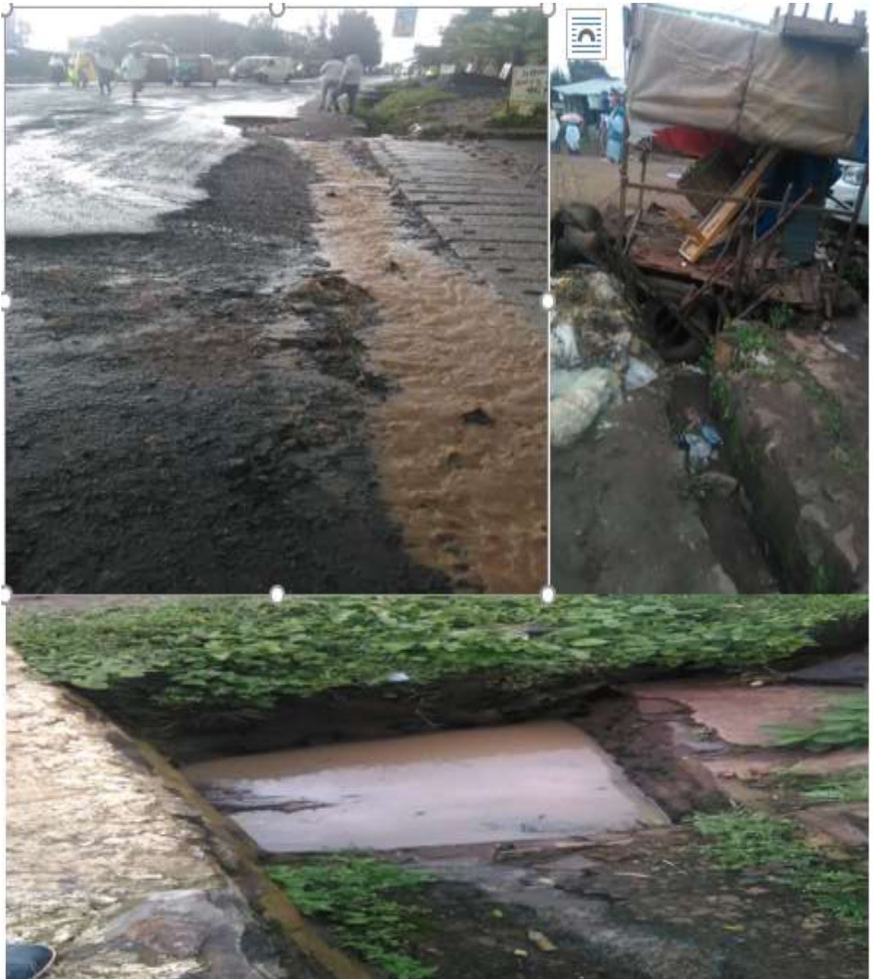
Figure 4.18. Improper drainage size ditch along the main road flooding (Fieldwork ,2017)
