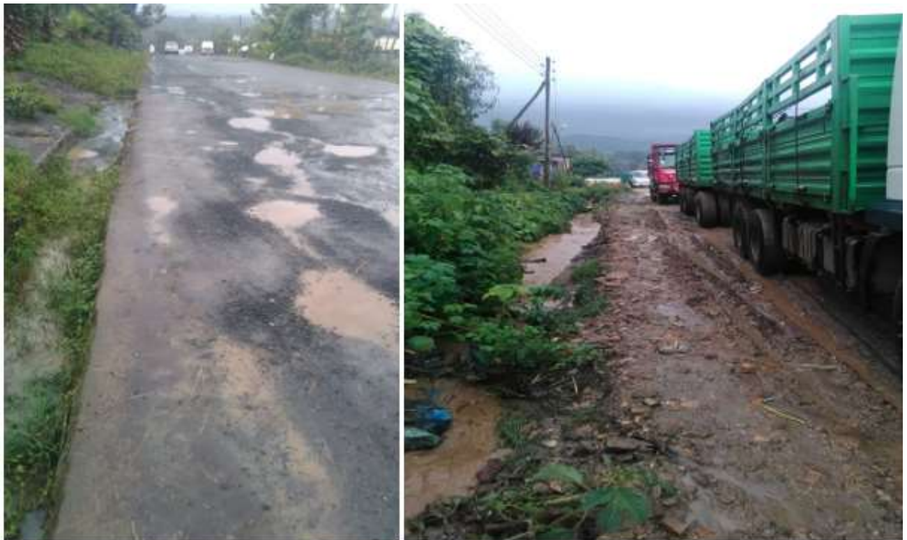
Figure 4.20. Crack road in Bure town street in Keble 2 (Fieldwork ,2017)
