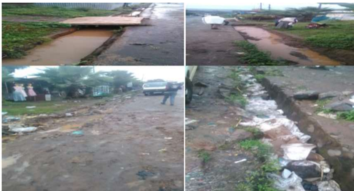
Figure 4.19: Open storm drainage system and improper slope (Fieldwork ,2017).
