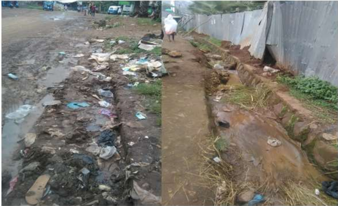
Figure 4.16 Blocked drainage network by sediment loading in Bure town (Fieldwork ,2017).
