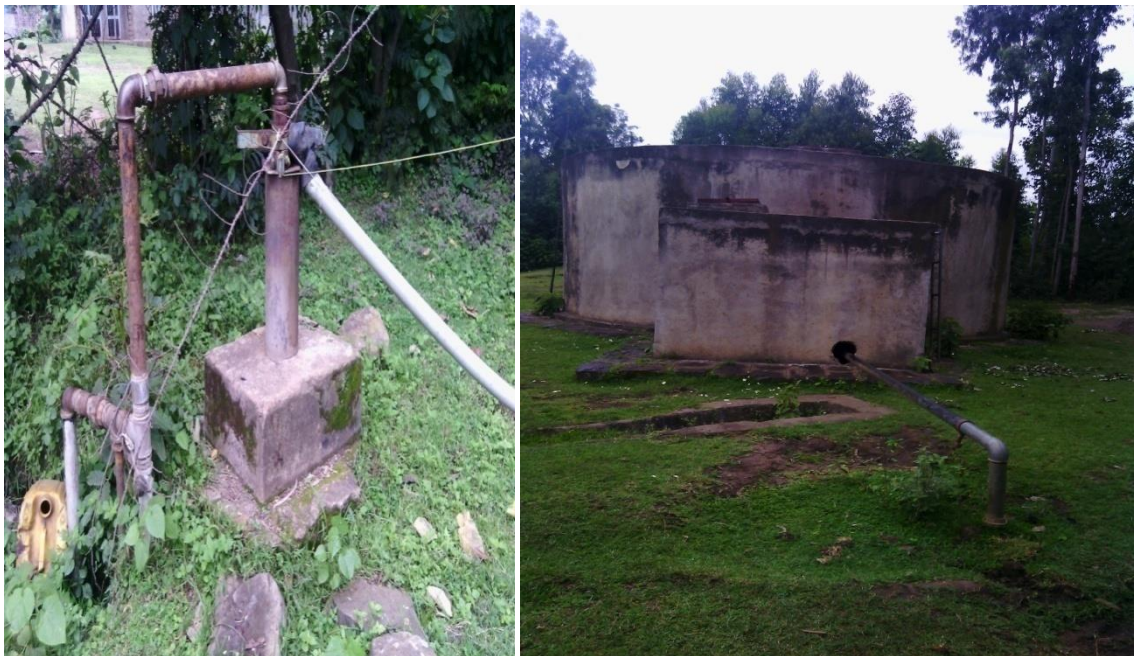
Figure 4.2 Faate BH and it's 100 m 3 reservoir
