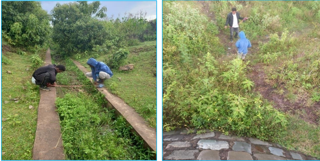
Figure 4.3 grass and silt accumulation
