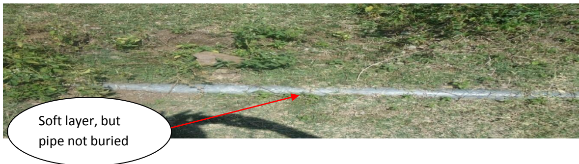
Figure 4.4 Poor installation of pipe line (Photo by: Researcher 15/ 9/ 2015)
