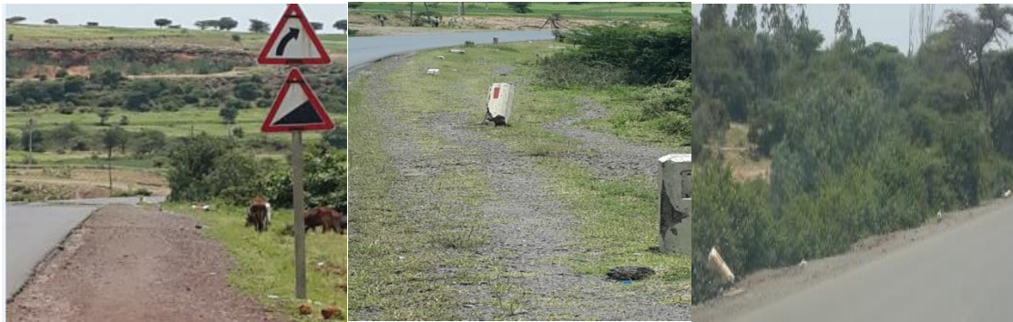
Photos 4.13: Gradient sign and guide post problem
