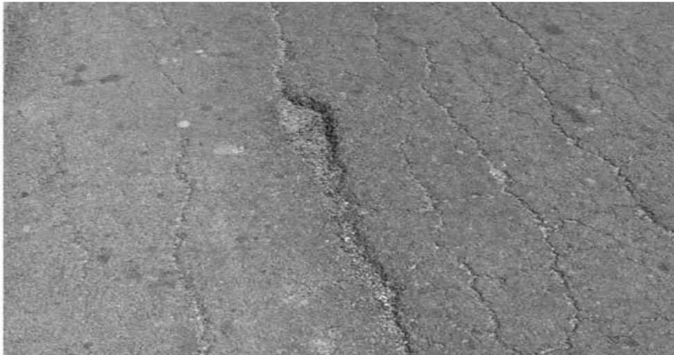
Figure .2.2. Longitudinal Cracking
