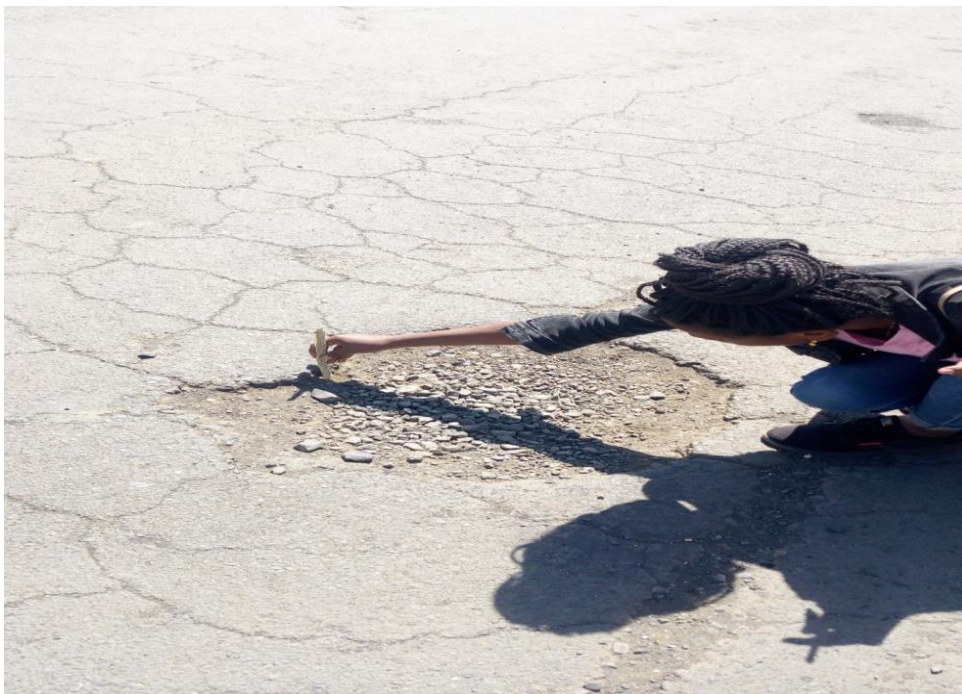
Cracking showing the potholes (Goro Sole in front of Construction Company)
