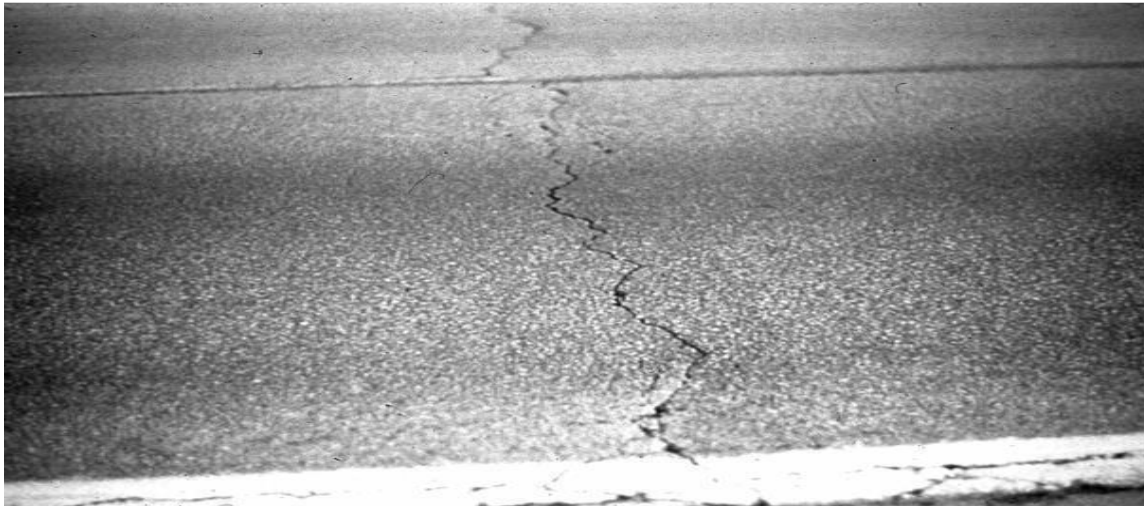
Figure . 2. 3. Transverse crack
