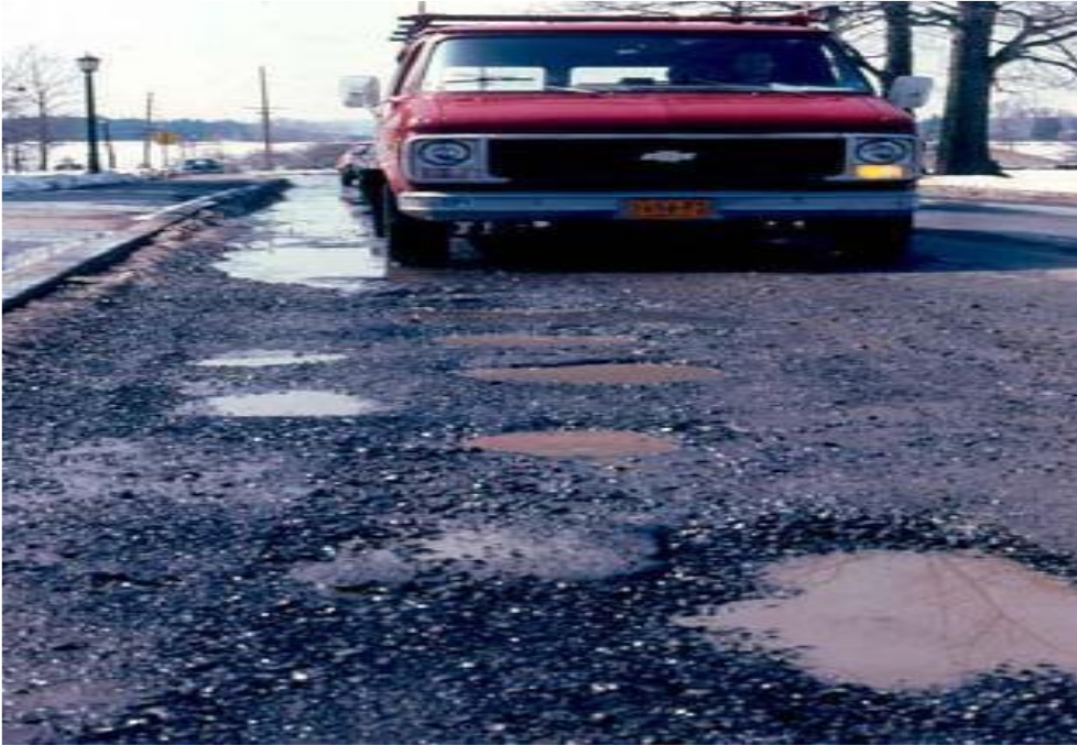
Figure .2. 4. Potholes caused by poor drainage
