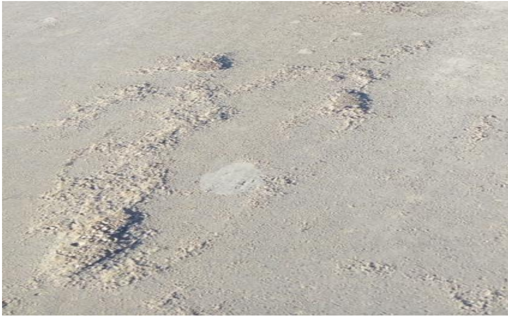
Fatigue cracking showing the beginning of a pothole (GUDER-GORO SOLE)
