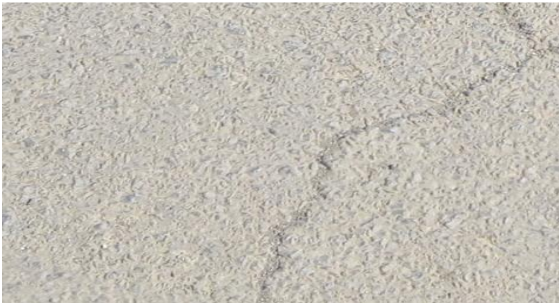
Transverse crack (GUDER)
