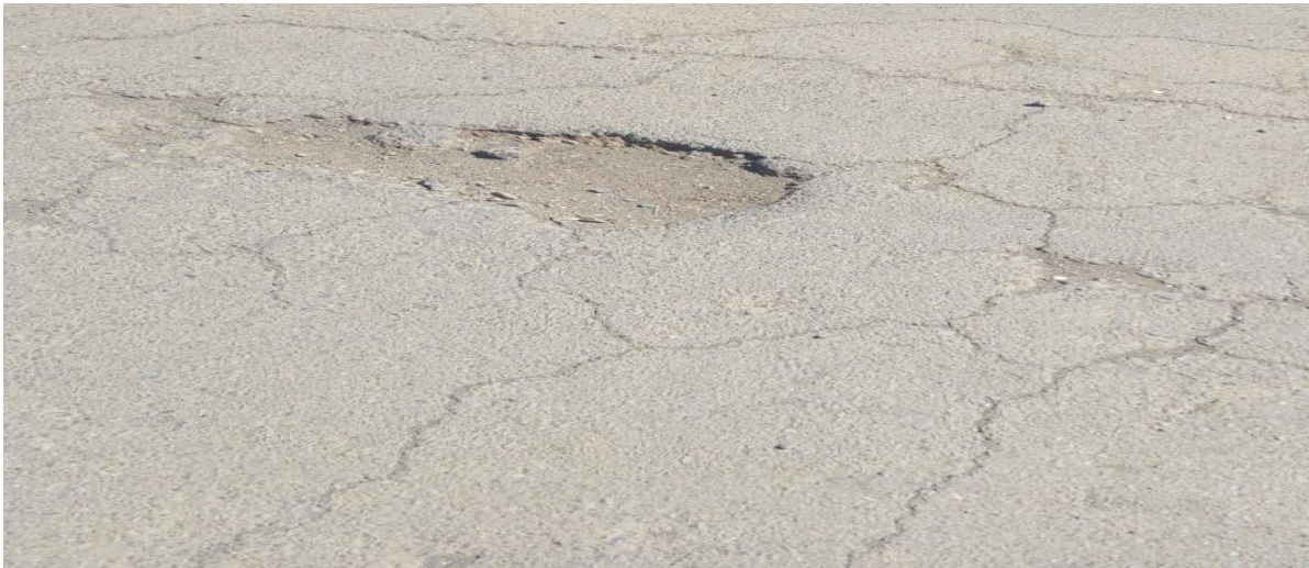
Pothole as a result of fatigue cracking(BABICH -GEDO)
