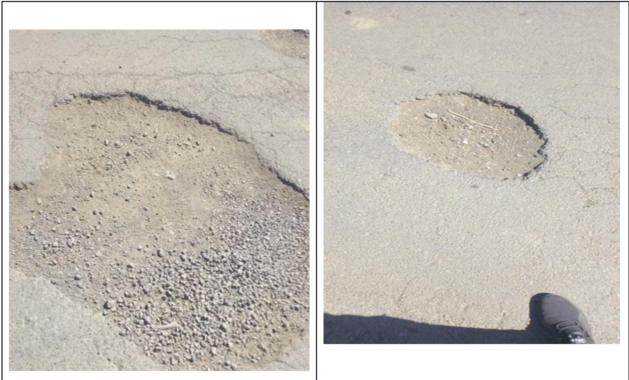
Pothole on a residential road after heavy rains(BABICH -GEDO)
