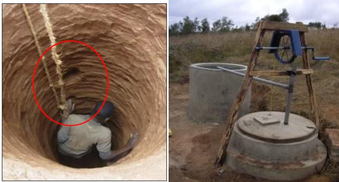
Figure 1: Photo of Traditional Hand Dug Well fitted with rope Pumps
