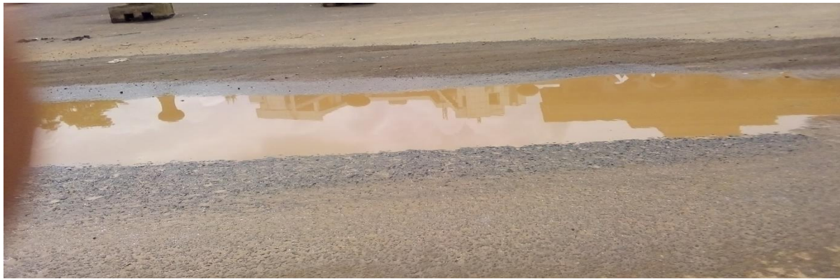
Figure 1. 1. Sleeping water along road side due to drainage problem [Photo taken by researcher on July, 2022 with smart phone]
