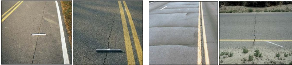
Wheel path cracking
