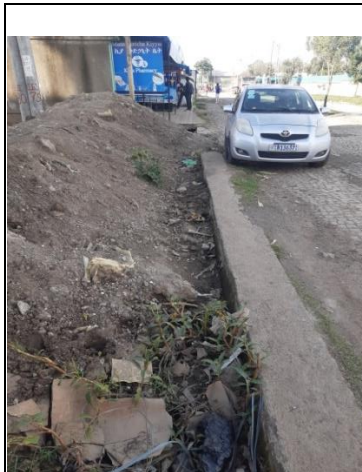
Drainage Chamfer not receiving Surface drains and ditch filled with sediment
