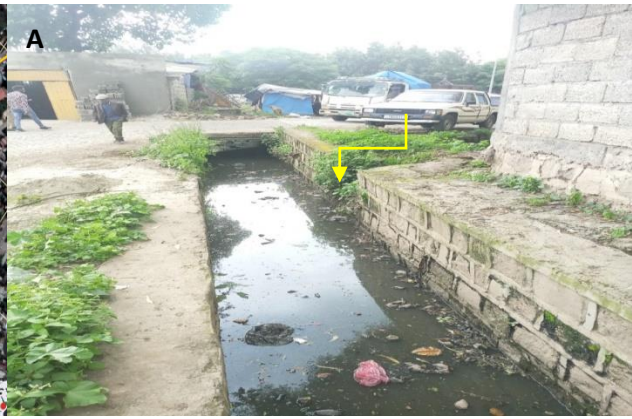
Blocked to prevent backflow
