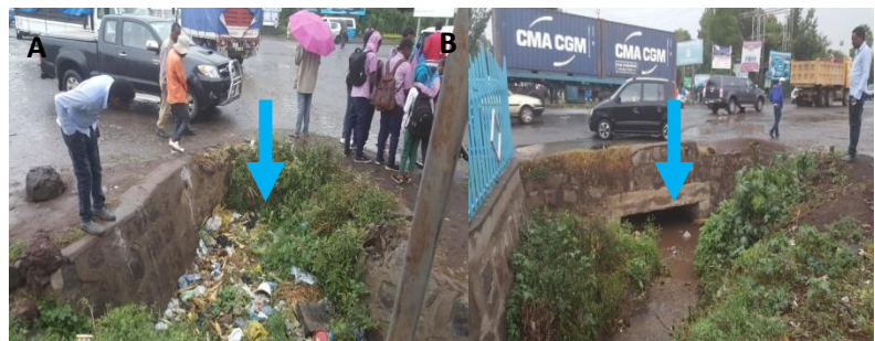
Inlet of pipe culvert blocked with solid waste.
