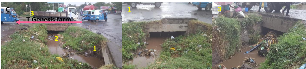
Culvert filled with solid waste and grasses
