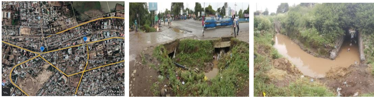
Location of structures Drainage filled with solid waste Drainage with L turn Figure 4. 13: Zikuala catchment drainage structures condition.
