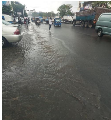
Flood flowing on the main road (no side drains)
