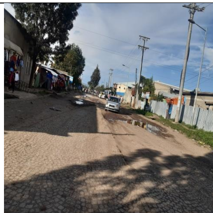
Defomed Cobblestone road by Flood detention of the surface
