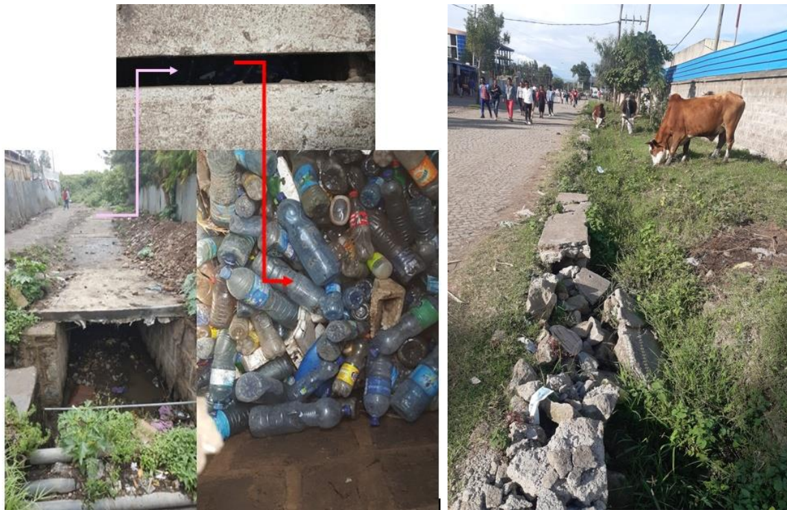
Accumulated plastic waste concealed by slab cover Figure 4. 16: Conditions of drainage structures.
