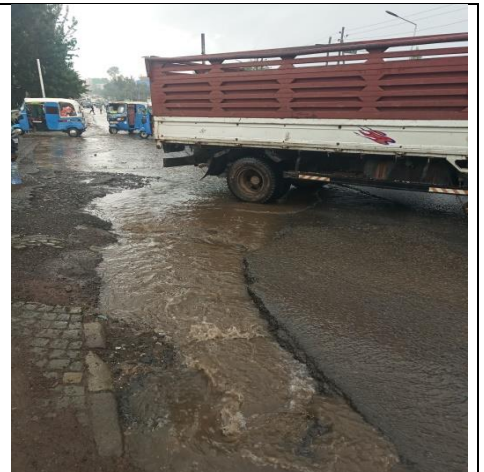
Road started eroding by surface runoff
