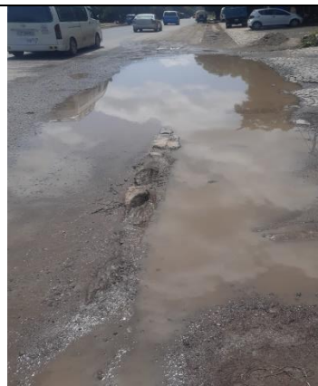
Improper connection of both drainage and road
