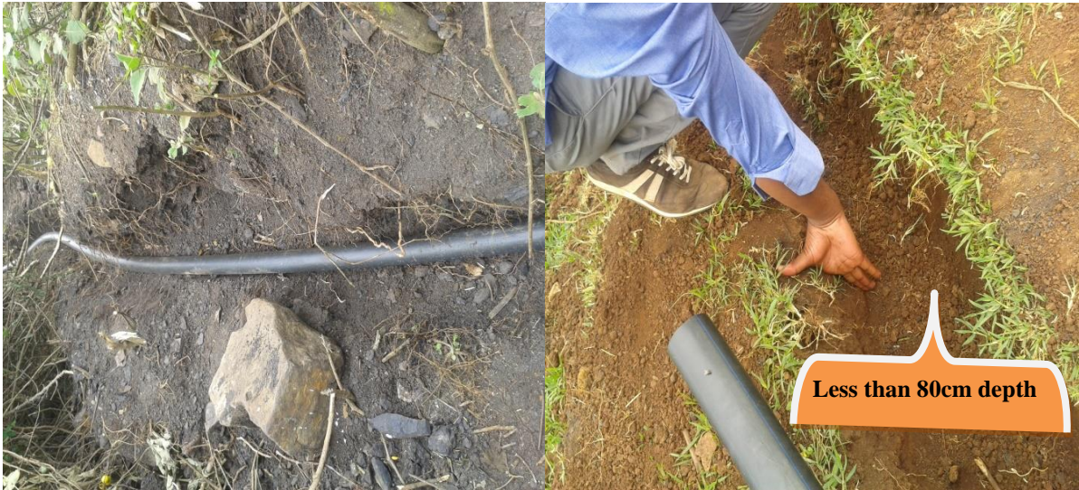
Figure 17 Pipe Trench excavation could not considered standards
