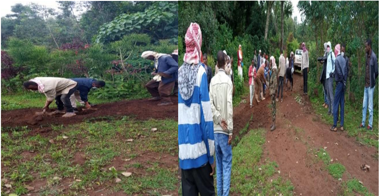
Figure 16 Community not properly coordinated during trench excavation
