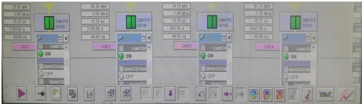
Figure 2.4 GG2 SCADA system displayed the power generated for each unit
