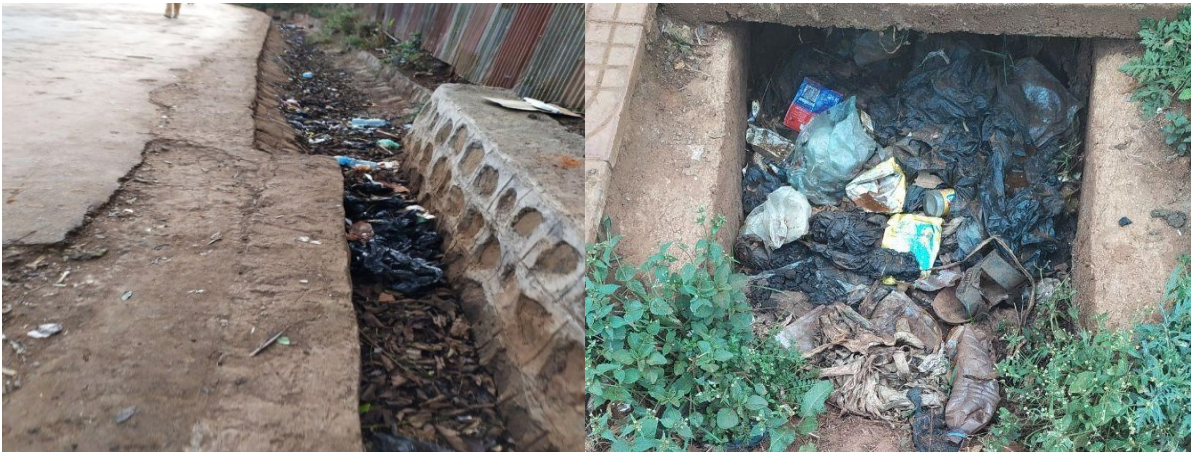
Figure 4. 8: Improperly designed drainage system
