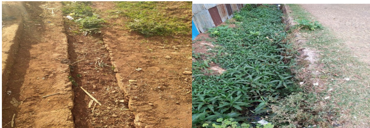
Figure 4. 5: An open channel type clogged by grass and silt
