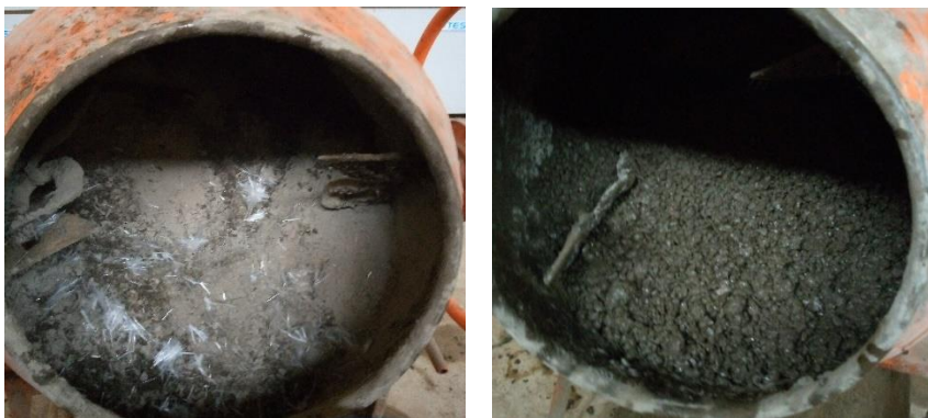
Figure E-3: Photos captured during the dry mix and wet concrete in a mixer.
