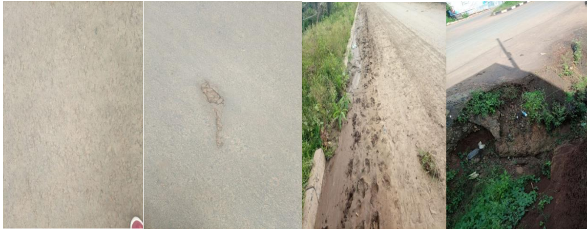
Figure 3-7 Distresses along Tarcha-Turi segment
