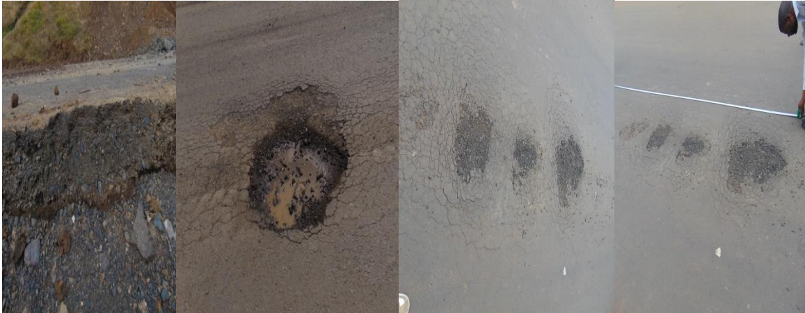
Figure 3-9 Distresses observed in Tulema-Gesa section
