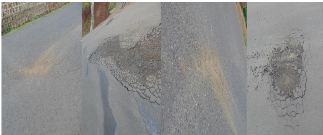
Figure 3-10 Distresses in Gesa-Elabqacho road segment
