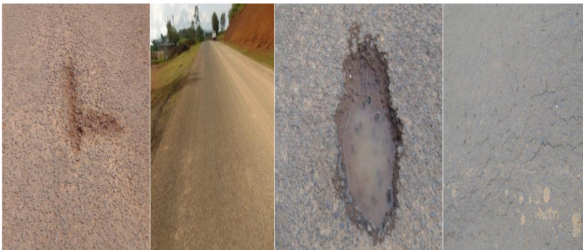
Figure 3-8 Distresses in Waka-Tulema road segment
