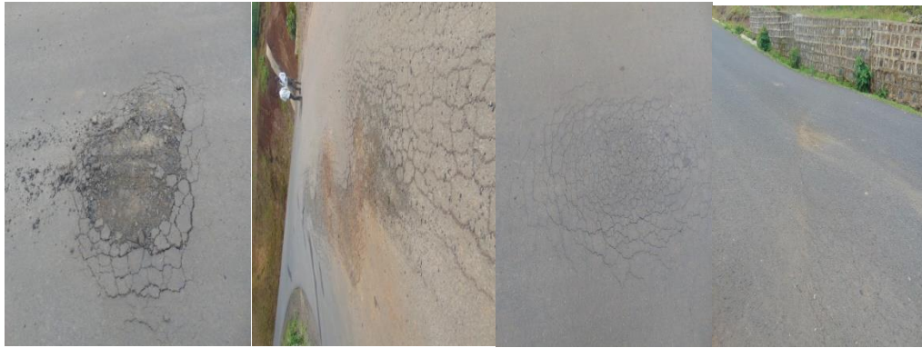
Figure 3-11 Distresses in Elabacho-Yalo road segment
