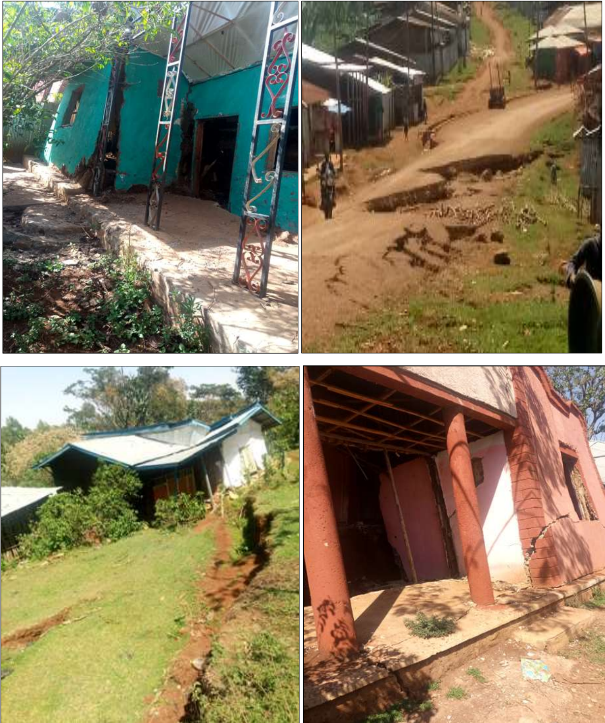
Figure 3.3 Cracks observed on the earth mass and Effects on residential houses.
