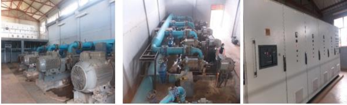
Figure 3. 7 New WTP pump house and switch board (Photo taken by the researcher)
