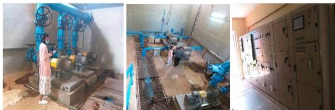
Figure 3. 6 Old WTP pump house and switch board (Photo taken by the researcher)
