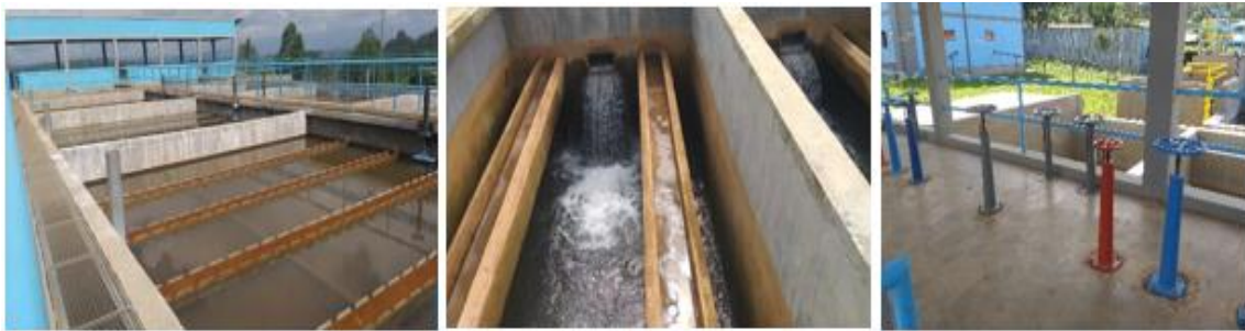
Figure 3. 8 a) Sedimentation, b) sand filtration, c) control get valves of new WTP (Photo taken by the researcher)
